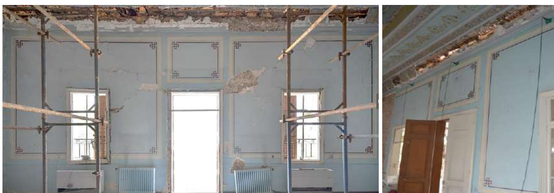
Damage assessment and mapping
