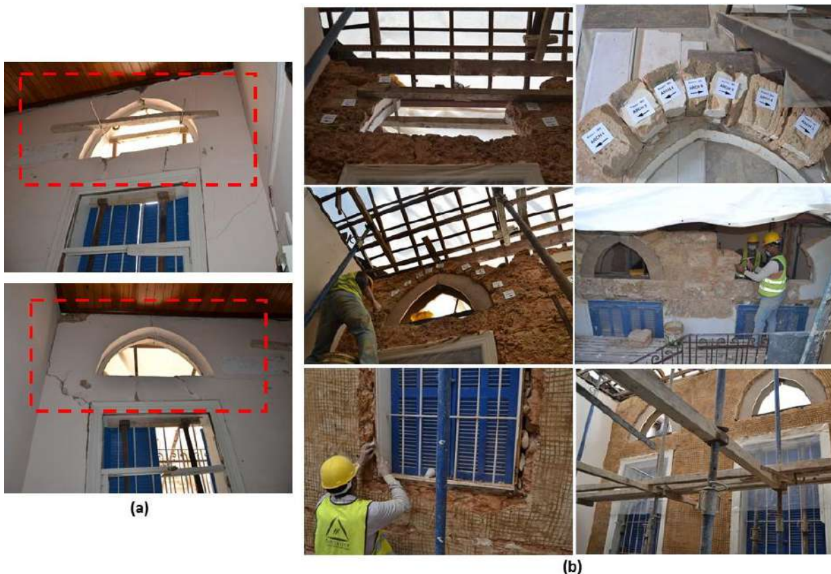
(a)- Deformed wall above arches, (b)- Wall consolidation: partial dismantling, remounting, deep repointing and plastering
