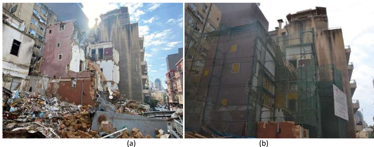
Exterior view of the building, (a)- Upon the blast, (b)- After stabilization works
