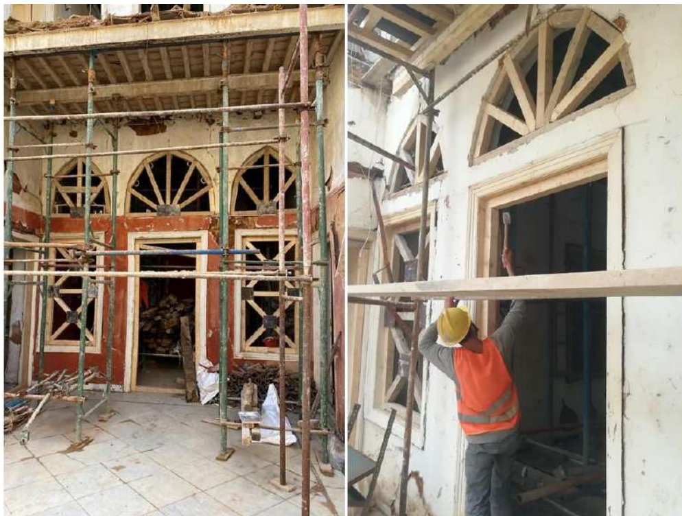
Propping and Strangling systems at all rooms
